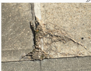
Stress Damaged Corners - Page 8
