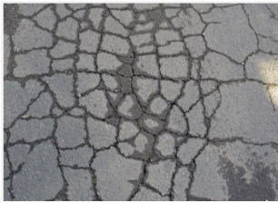
Shrinkage Cracking - Page 7
