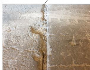
Failed Slab & Joint Edges - Pages 8 & 9
