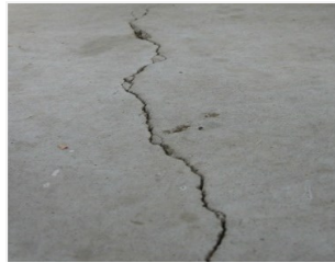
Structural Crack - Page 6
