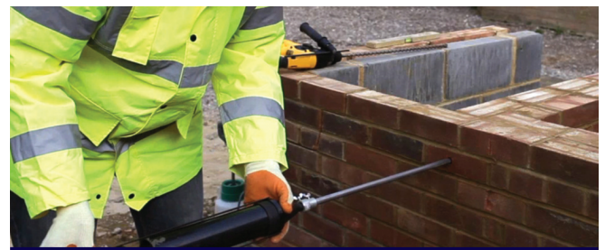
Inserting the grout-filled pinning nozzle, containing the CemTie, into the clearance hole
